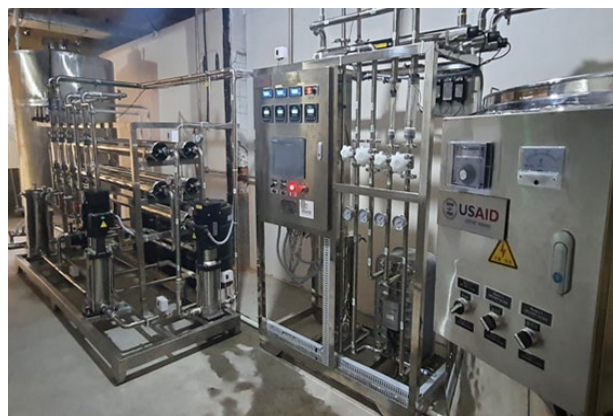
PQM+ supported water treatment system improvement at Nepal Manufacturer 6.
